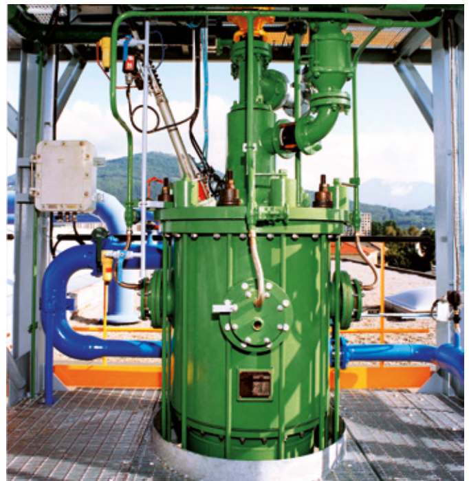
↑ Top of combustion chamber and ignition system
